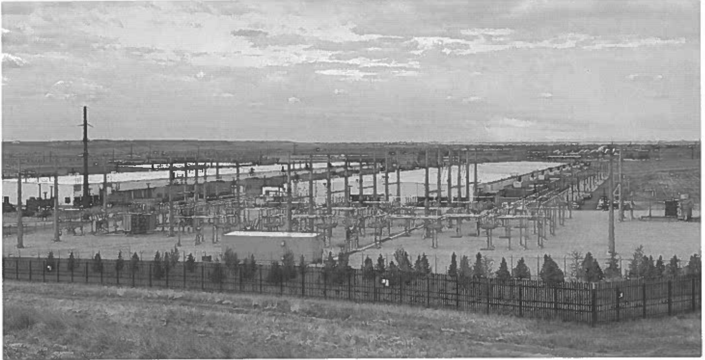
Microsoft's data center in the Cheyenne Business Parkway business park in east Cheyenne. (Greg Johnson, Cowboy State Daily)
